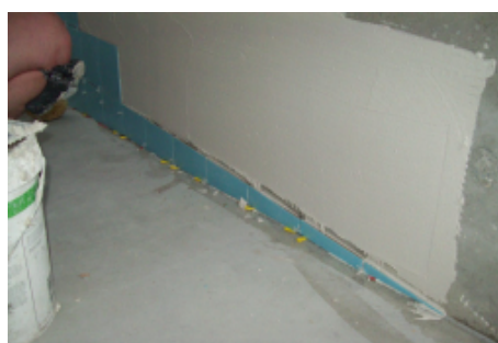
Figure 8 Sharp tile ends should be avoided within pool tanks
