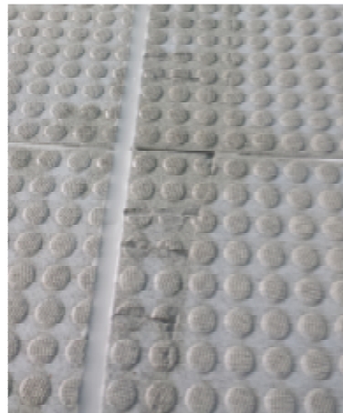
Figure 7. Excessive movement causing cracking immediately adjacent to a movement control joint
