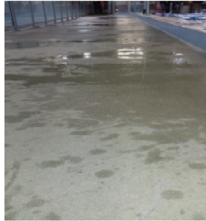
Figure 3 Inadequate drainage greatly increases cleaning demand and slip potential
