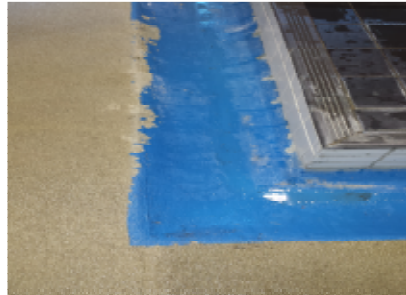
Figure 4 Open channels, even when clearly marked, create tripping hazards
