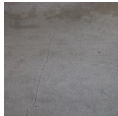
Figure 6. Cracking in a resin surface as a result of no movement control joints
