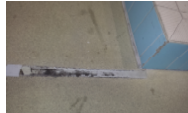
Figure 5. Allowance for movement and correct sealant selection is critical. Note damage to exposed tile edges also
