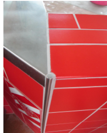
Figure 9. Thoughtfully placed edge protection to exposed corners limits surface damage
